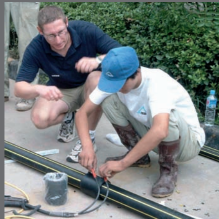
Demonstration of an electrofusion process. No questions remain unanswered when there is training on the construction site.
